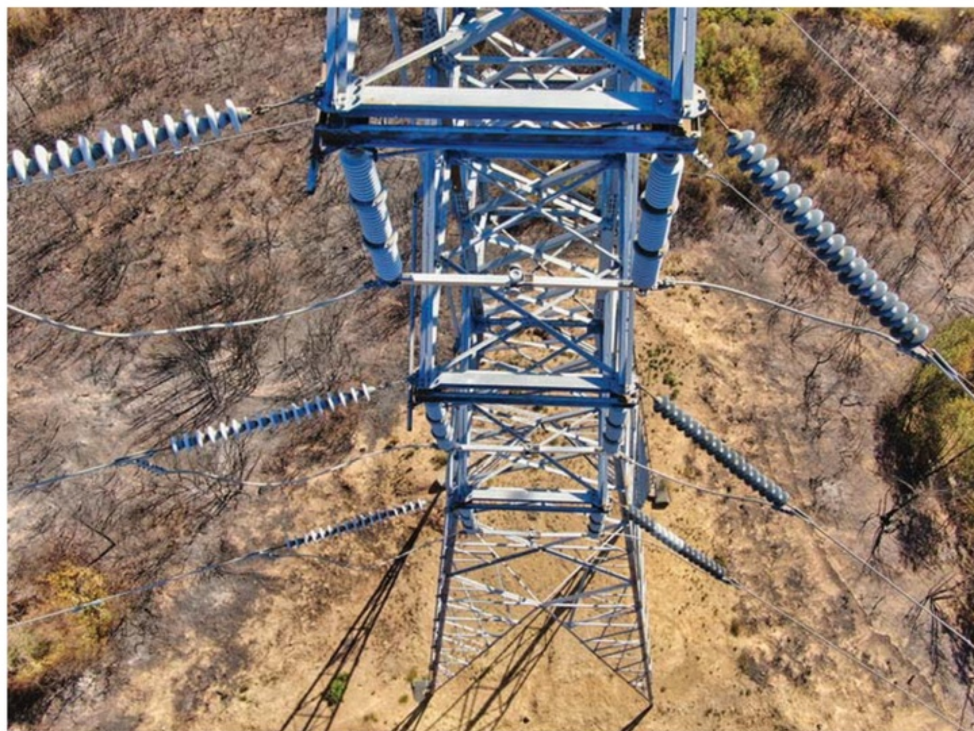
Overhead view of metal transmission tower surrounded by scorched earth. Photo by POWER Engineers.
