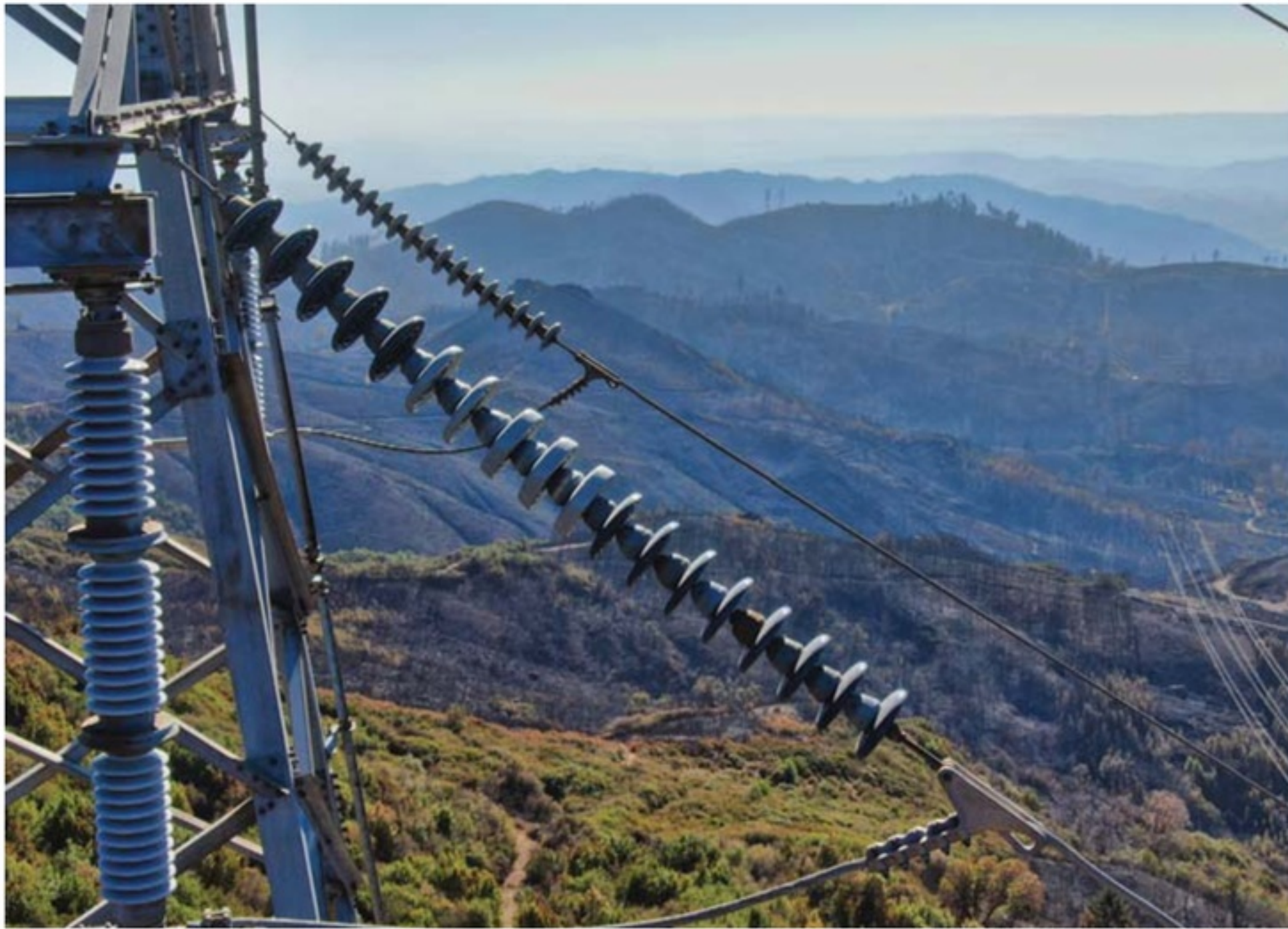
Metal transmission tower overlooks a fire scarred mountain. Photo by POWER Engineers.
