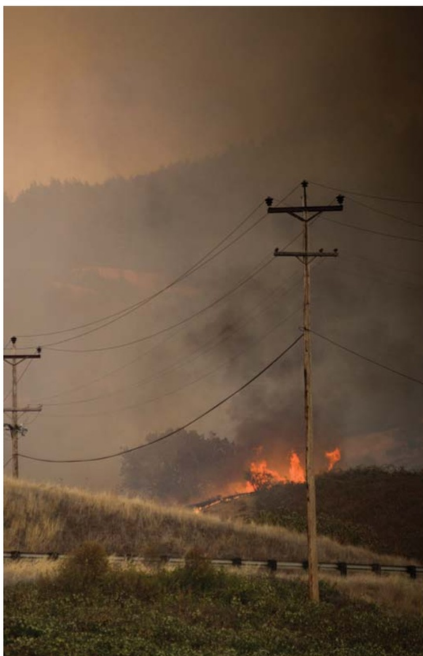
Wooden poles in the face of fire. Photo by POWER Engineers.
