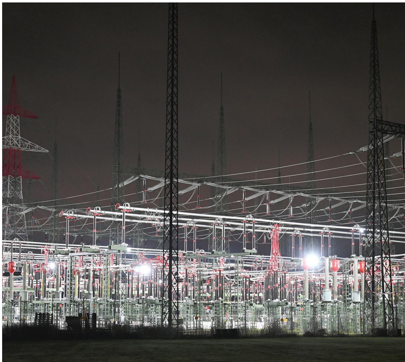
A substation in Austria at night. Utilities should take a calculated and educated approach to mitigations to find the most acceptable balance between security and cost. Photo 262839930 © Wolfgang Spitzbart | Dreamstime.com
